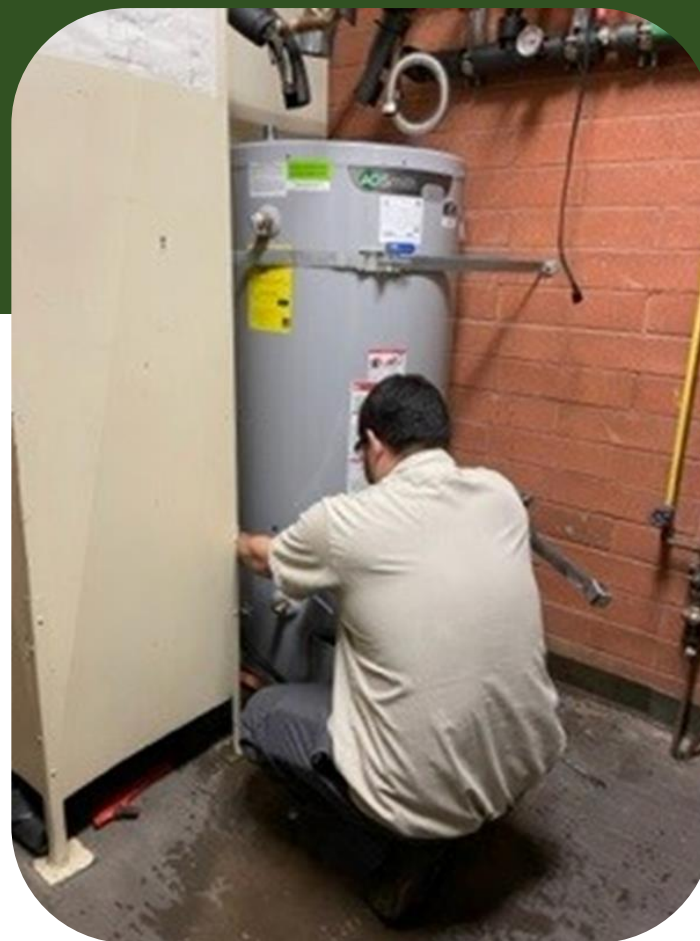
Cleaned and maintained ~30 city owned buildings, including maintenance of internal systems and devices
