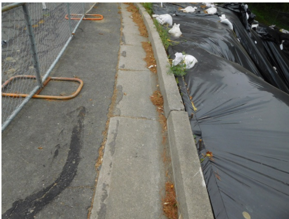
Photograph 17. Cracking and offset curb & gutter 5/24/23.
