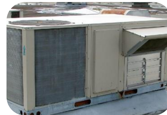
#36014 Processing Building Ventilation
