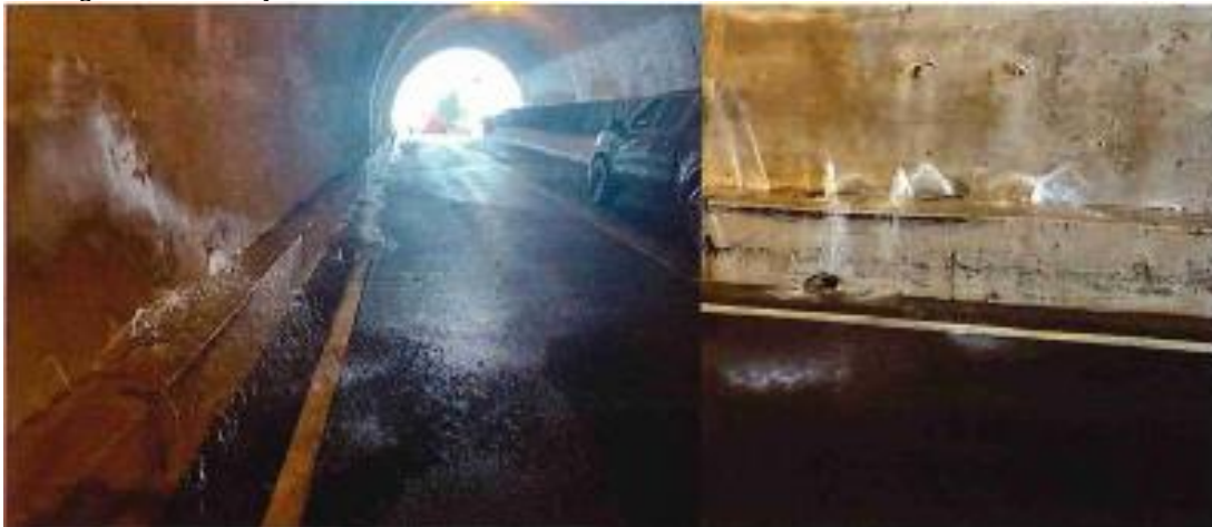
Image: First sanitary sewer overflow that occurred from the broken line that is encased in concrete
