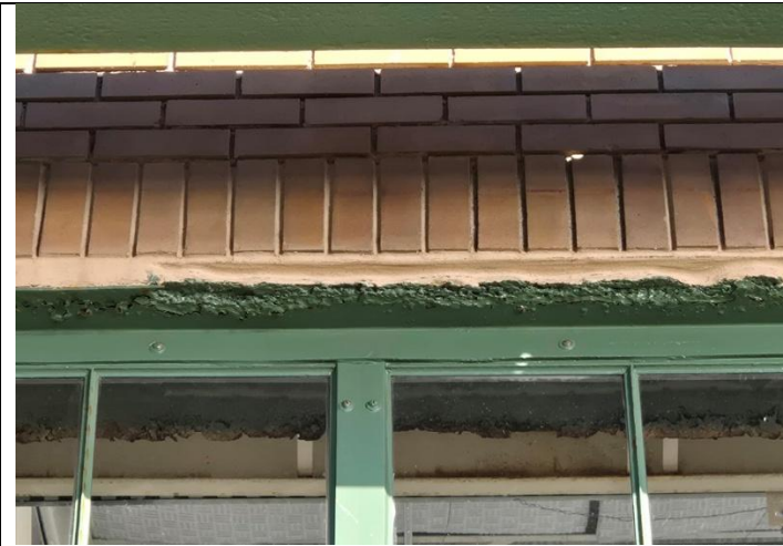
Figure 9. Corrosion and sectional loss of lintel, previously painted over
