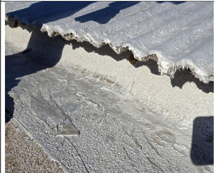
Figure 47. Steep-sloped coated transite roof panels at upper sawtooth roof
