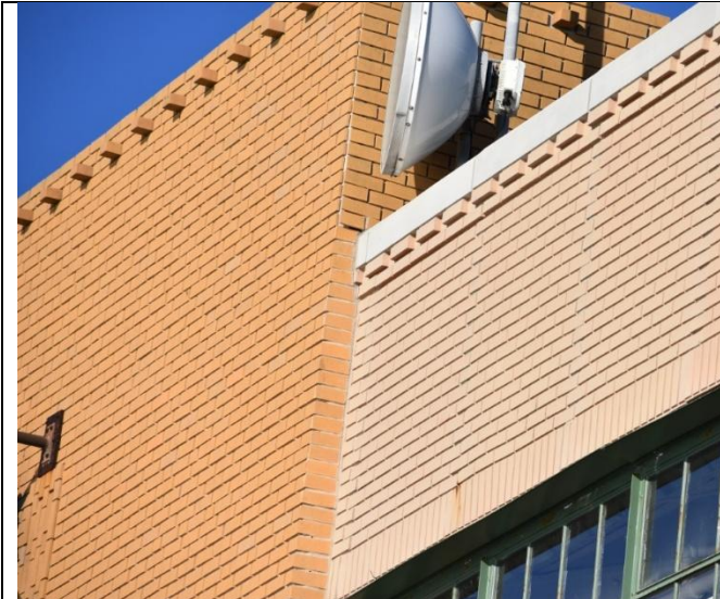
Figure 13. FRP/fiberglass panelized parapet assembly with adhered brick veneer; replacement for collapsed parapet in Loma Prieta earthquake
