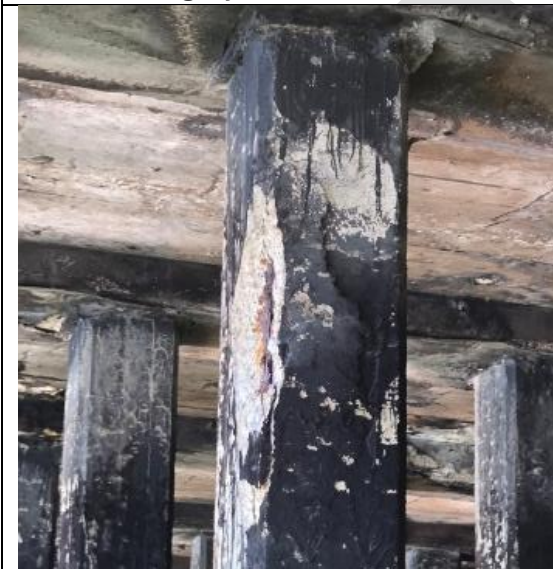
Figure 75. Significant spalling and sectional loss present, corroded reinforcing visible – Severe Defect Category
