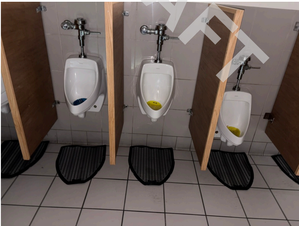
34 - Typical urinals in the men's restroom.
