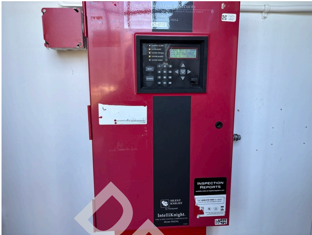
53 - Main fire alarm control panel located in the Main Building.
