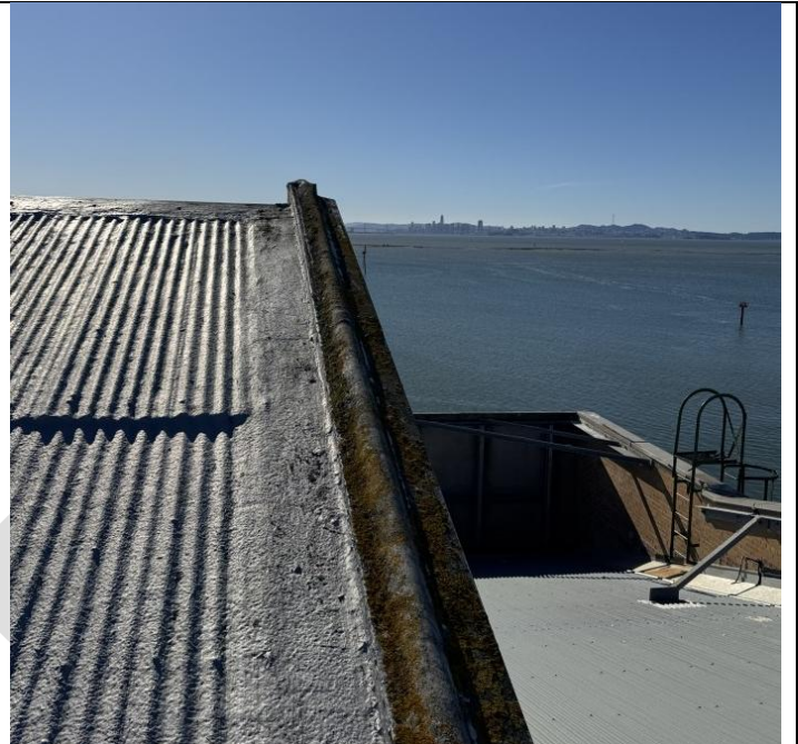
Figure 66. Expansion joint bellows at roof edge with organic matter
