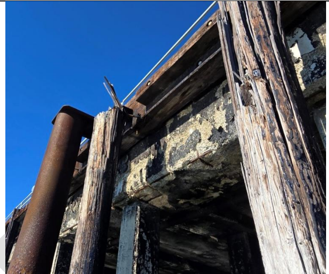
Figure 78. Deteriorated wooden pilings and corroded steel pilings
