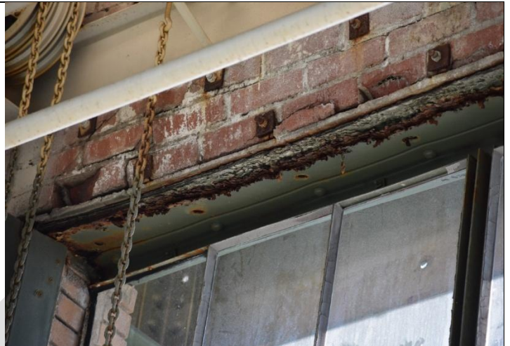
Figure 10. Significant corrosion and sectional loss of lintel as viewed from interior
