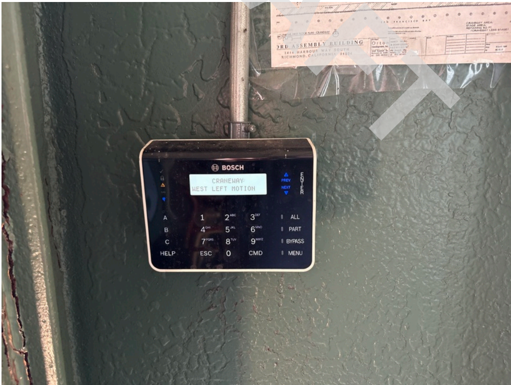
64 - Typical security alarm station in the Craneway Pavilion.
