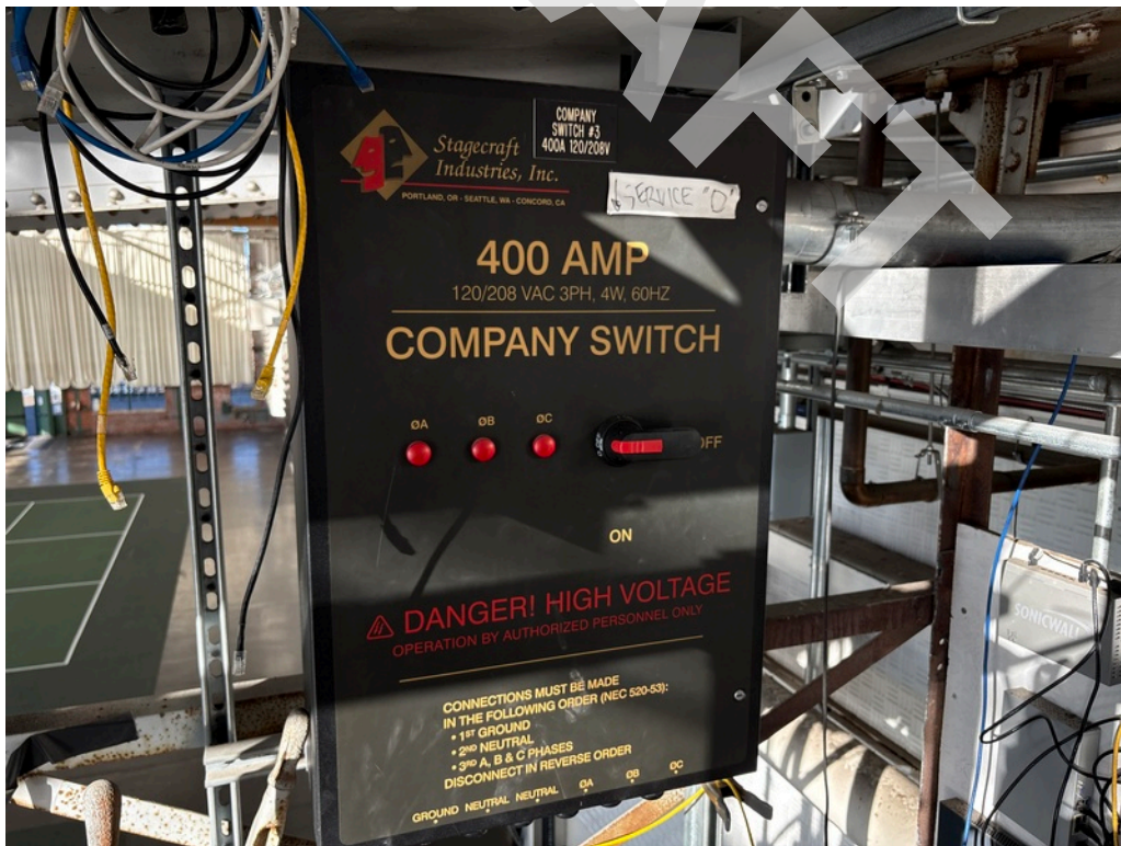
42 - One of two A/V special electrical panels. This is located on the west beam crane's operator's station.
