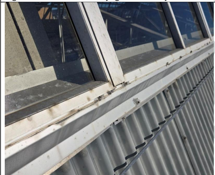
Figure 63. Condensation gutter at inside of skylight frame. Minor aluminum surface corrosion present on exterior surface
