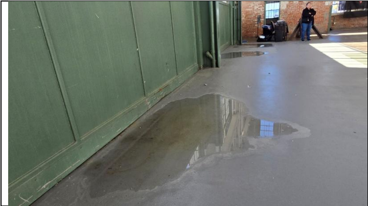
Figure 33. Ponding at base of painted overhead door on south elevation
