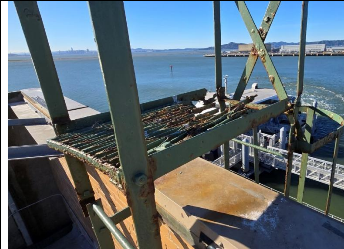
Figure 45. Significantly corroded ladder with sectional loss
