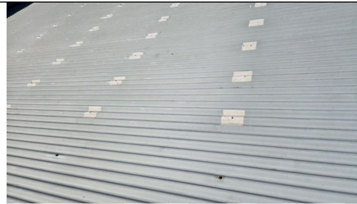
Figure 51. Localized liquid flashing/sealant over fastener penetrations; some corroded fasteners present
