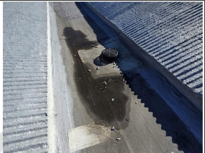
Figure 58. Ponding water near area drains
