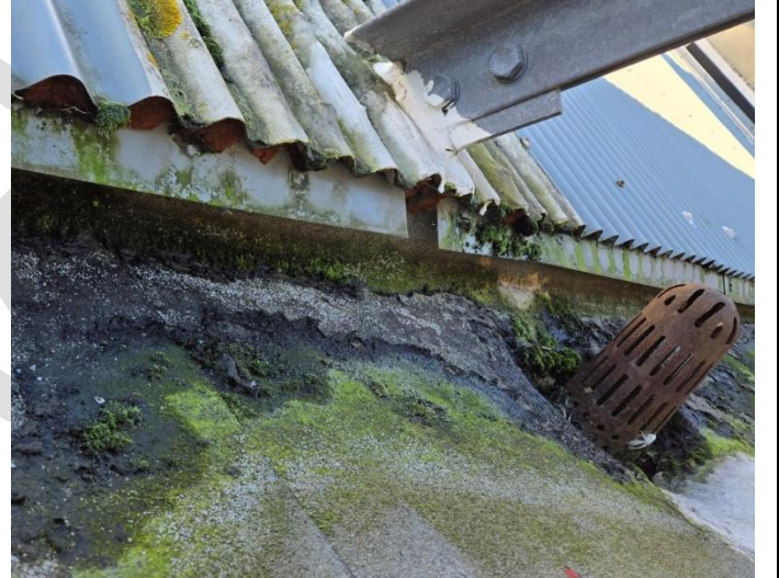
Figure 60. Organic material growth and ponding at low-spot near drains
