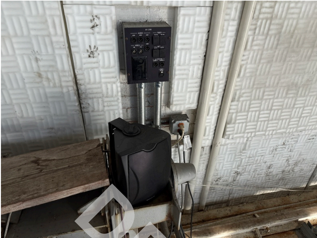
51 - Typical A/V connection panel.
