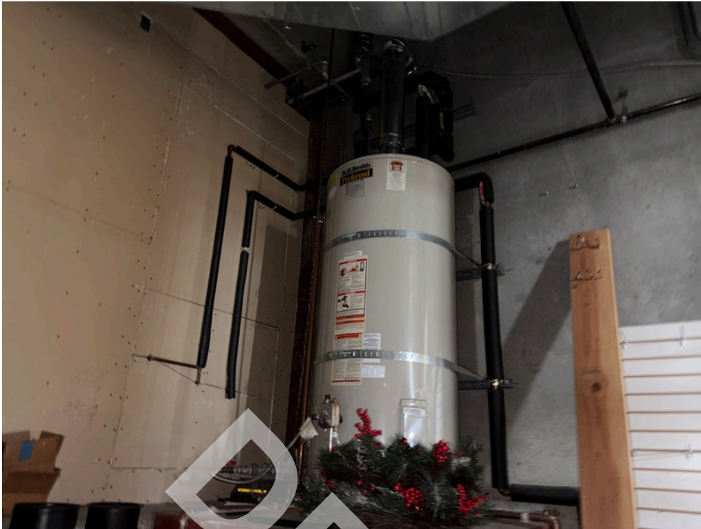
37 - Domestic water heater for the service kitchen in the adjacent utility room.
