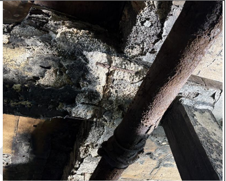
Figure 82. Spalling and sectional loss at underside of slab and beam, including corrosion of reinforcing steel
