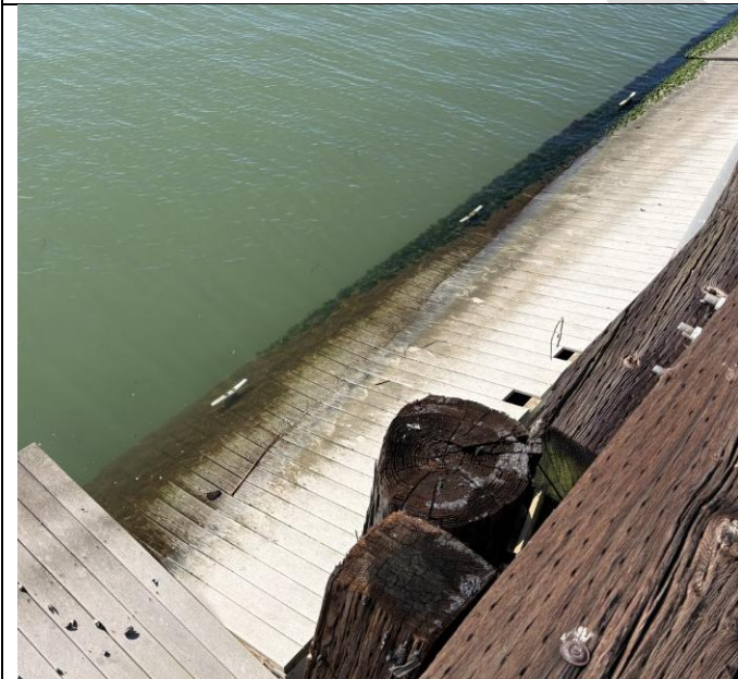
Figure 79. Partially submerged dock along southern elevation
