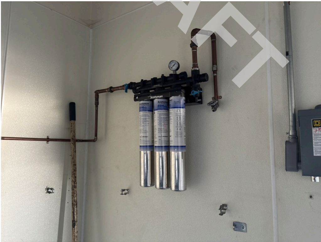
38 - One of two water filtration systems for the service kitchen.
