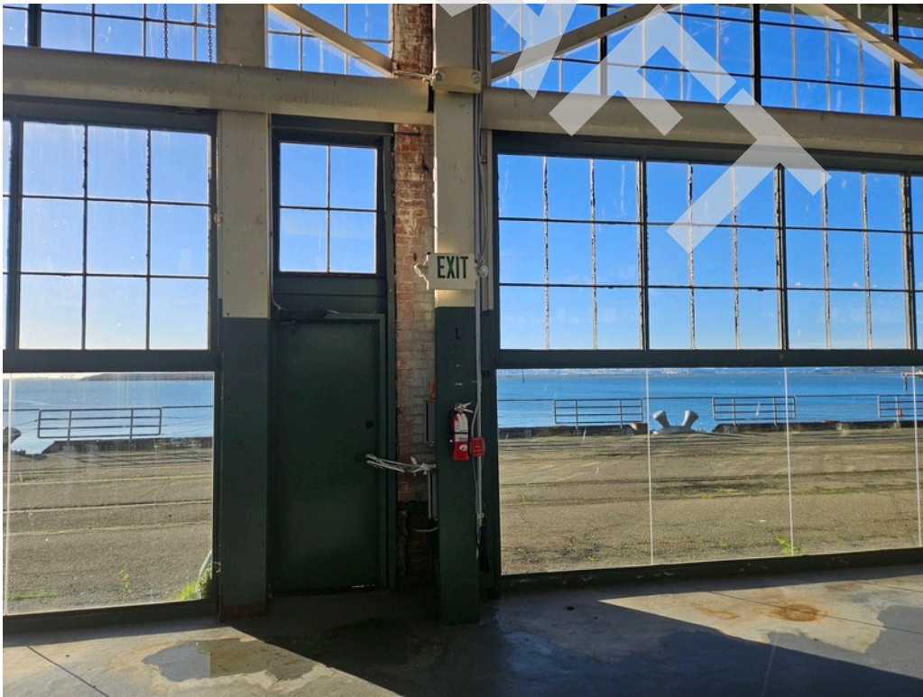
60 - Non-illuminated exit sign.
