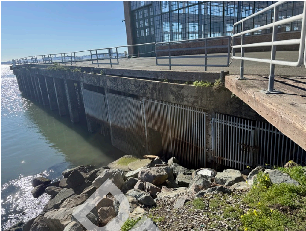
11 - Rusted and damaged metal picket fencing, located underneath the pier at the northeast corner of the site.
