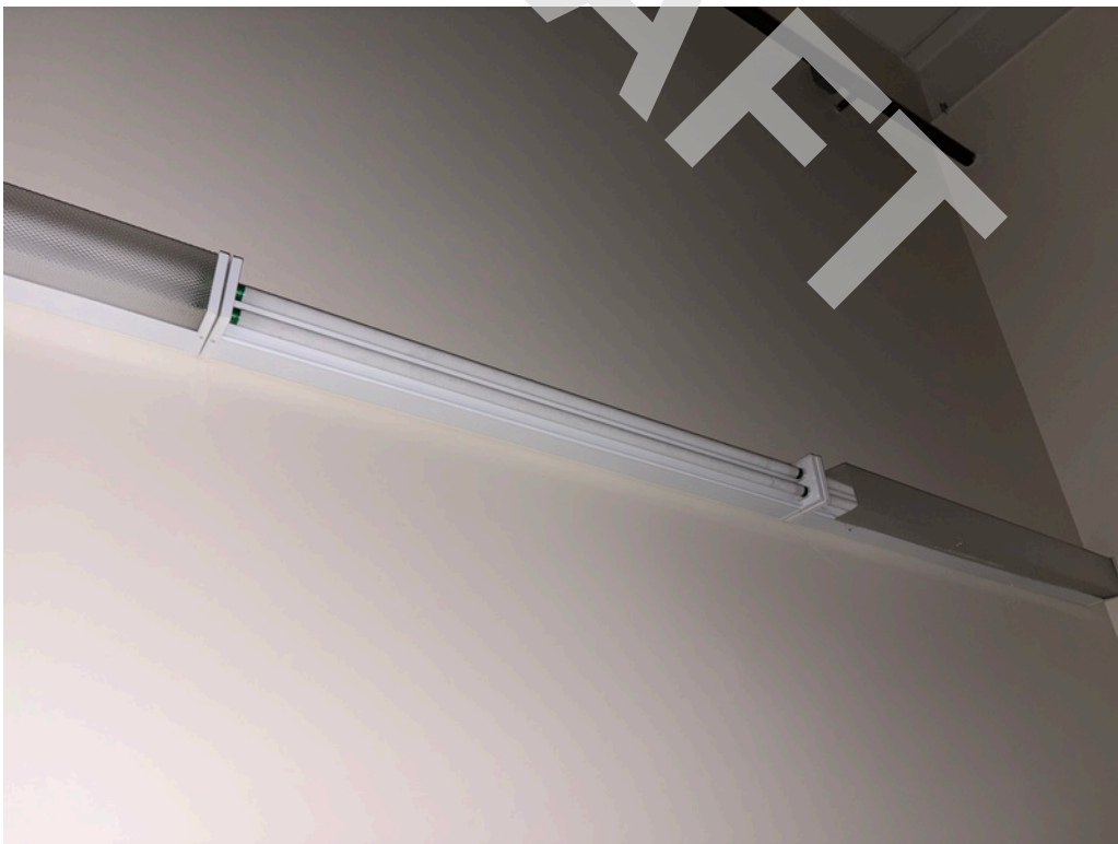
46 - Typical restroom light fixtures.
