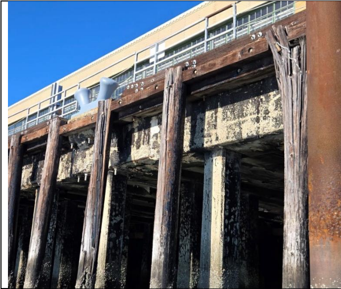
Figure 77. Deteriorated wooden pilings and corroded steel pilings
