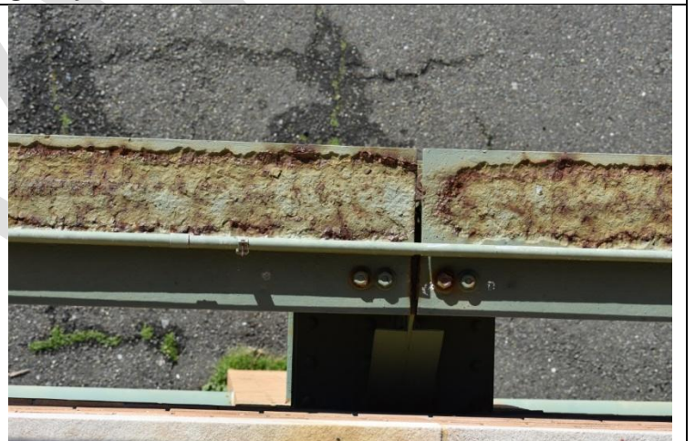
Figure 44. Surface corrosion and paint loss on steel gantry crane elements
