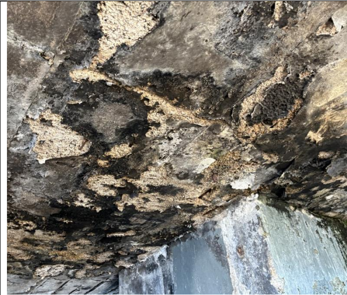
Figure 81. Example of delamination and spalling at underside of slab
