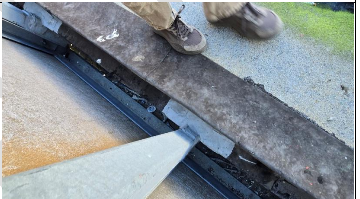
Figure 56. Transition from bituminuous membrane to EPDM membrane at roof edge condition adjacent to FRP/fiberglass parapet system
