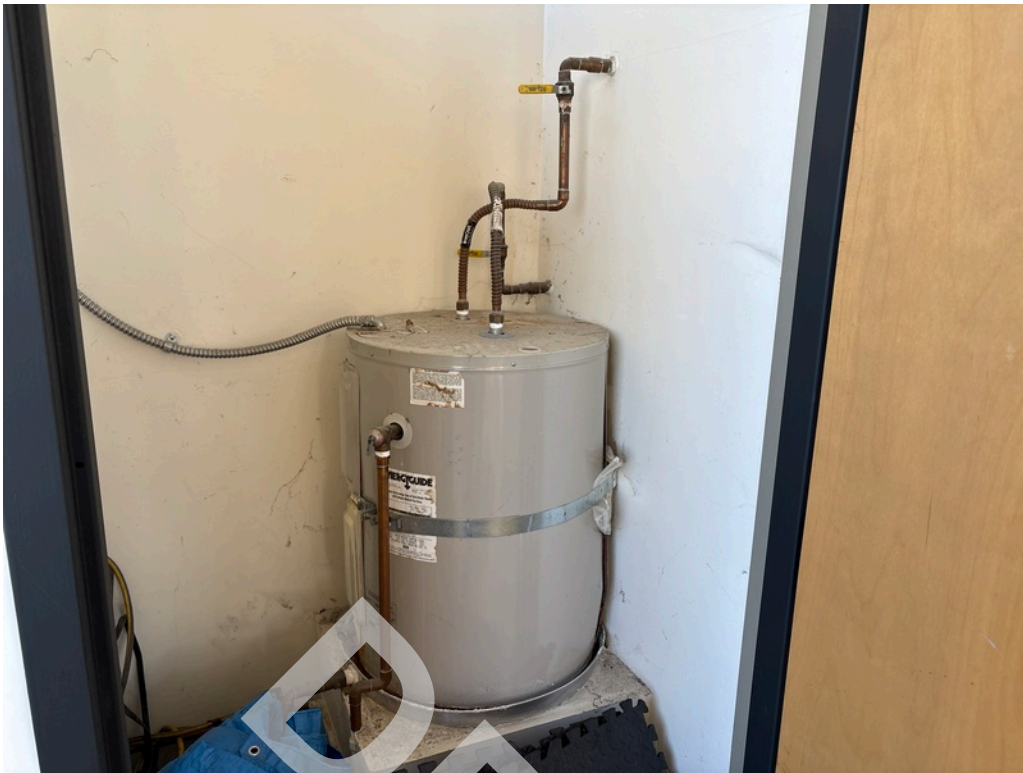
35 - Domestic water heater serving the restrooms.
