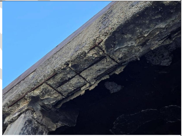
Figure 84. Spalling and sectional loss at perimeter beam, including corrosion of reinforcing steel
