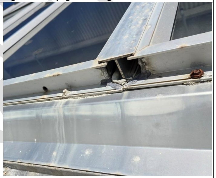
Figure 64. Drainage of vertical mullion. Corroded fasteners present at some locations
