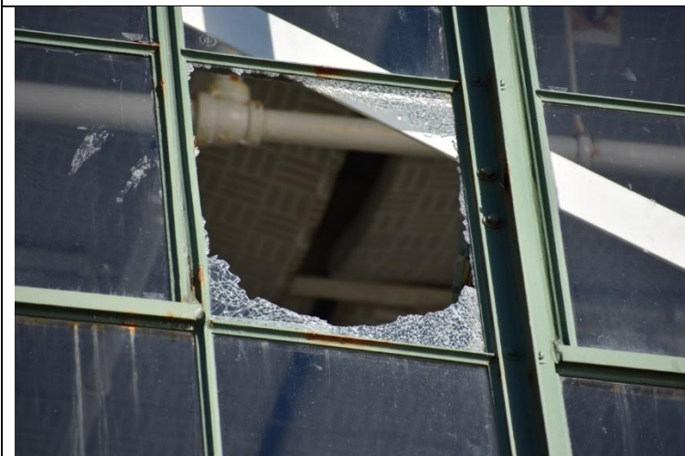
Figure 31. Shattered window pane
