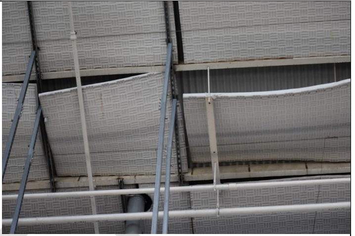
Figure 54. Acoustic insulation board detached from underside of metal roof deck
