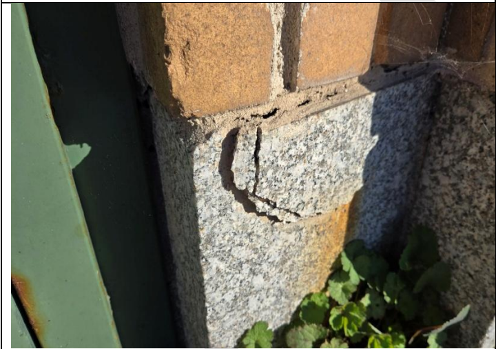
Figure 23. Spalling and corrosion staining at granite stone base
