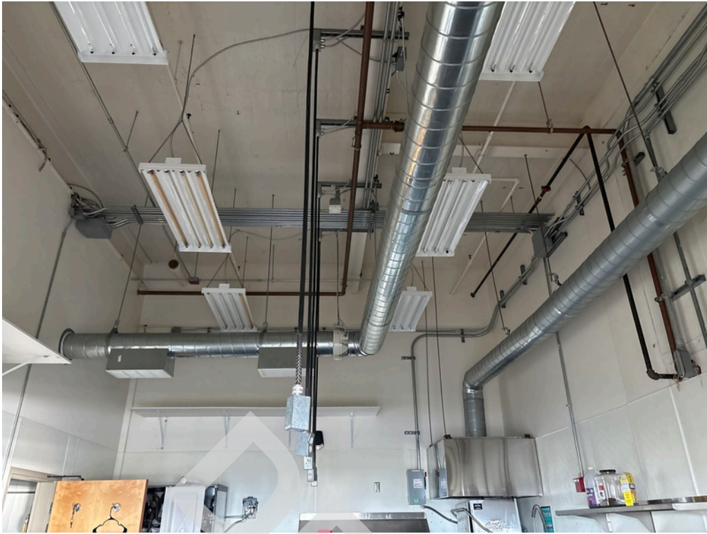
31 - Typical outside air supply ductwork and diffusers in the service kitchen.
