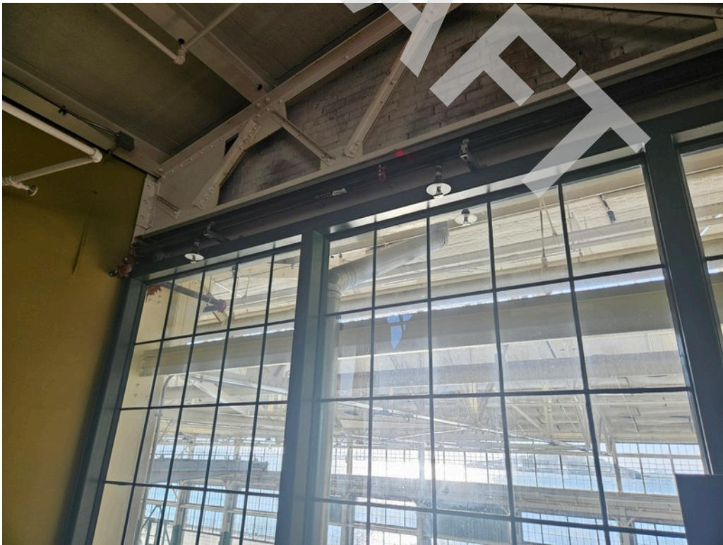
58 - Window sprinklers enhance fire separation between the areas.
