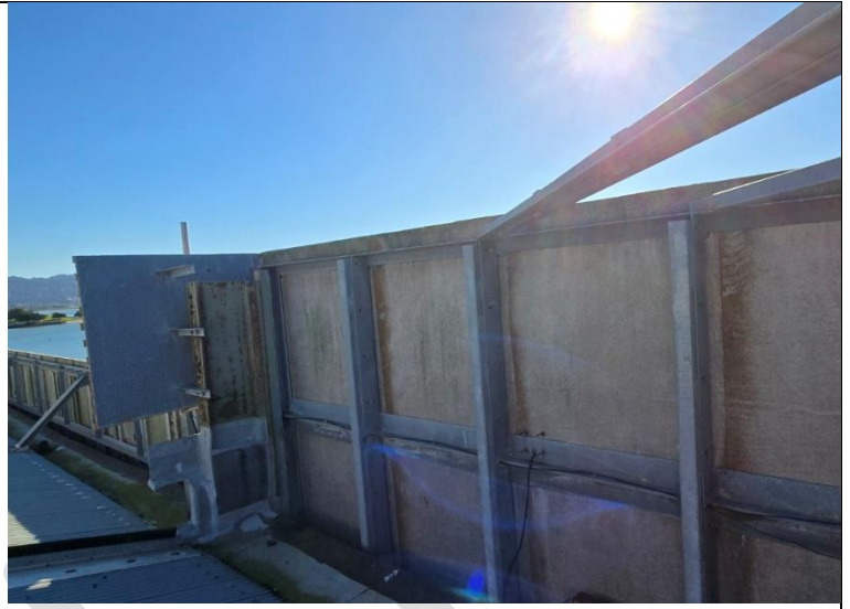
Figure 14. FRP/fiberglass panelized parapet assembly with adhered brick veneer; replacement for collapsed parapet in Loma Prieta earthquake
