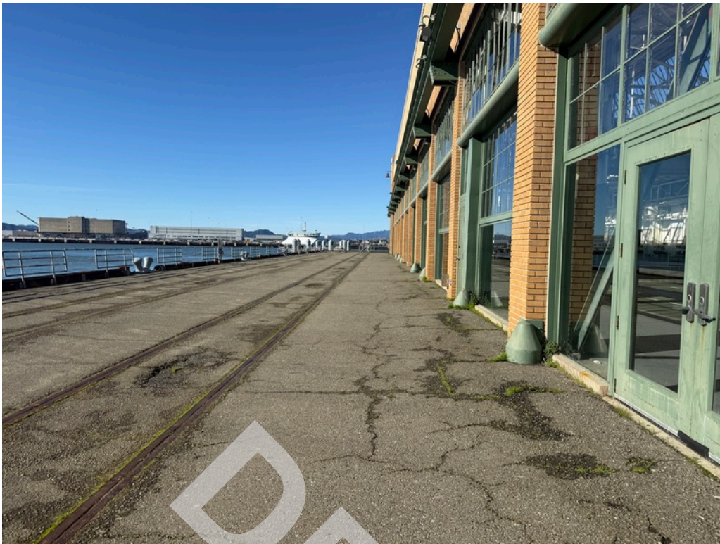
7 - Significant cracking and damage on the asphalt pavement along the south perimeter of the site.
