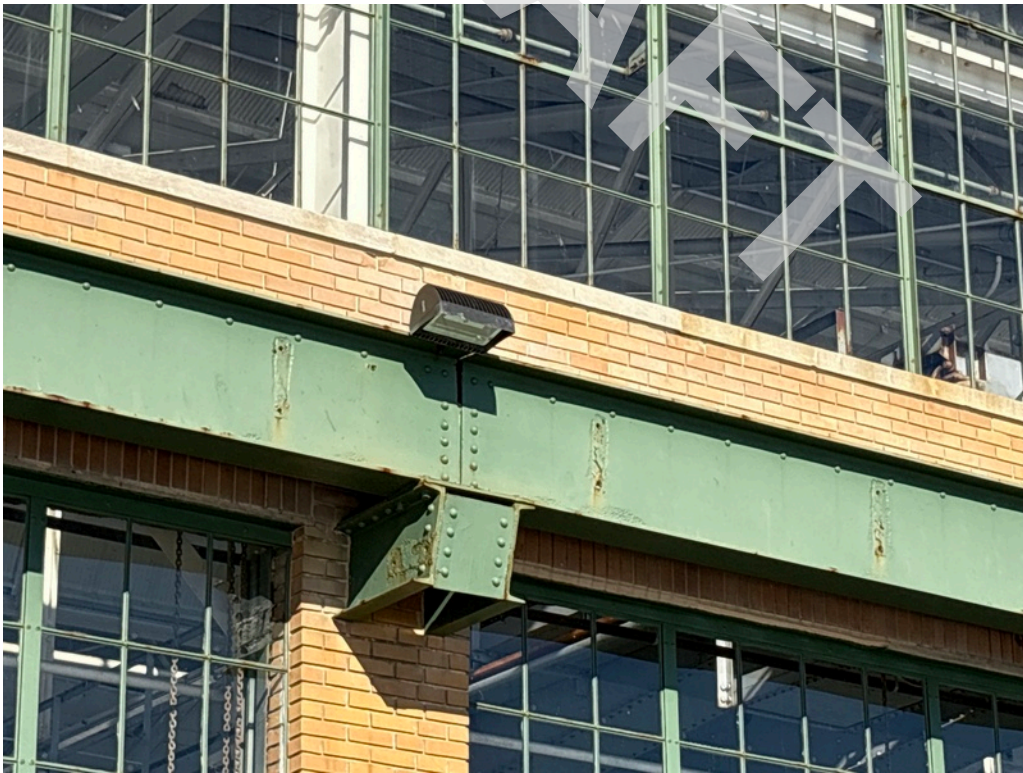
6 - Typical wall-mounted, exterior light fixture on the south elevation of the Craneway Pavilion.
