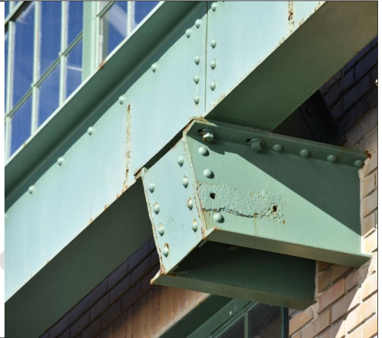
Figure 42. Surface corrosion and paint loss on steel gantry crane elements
