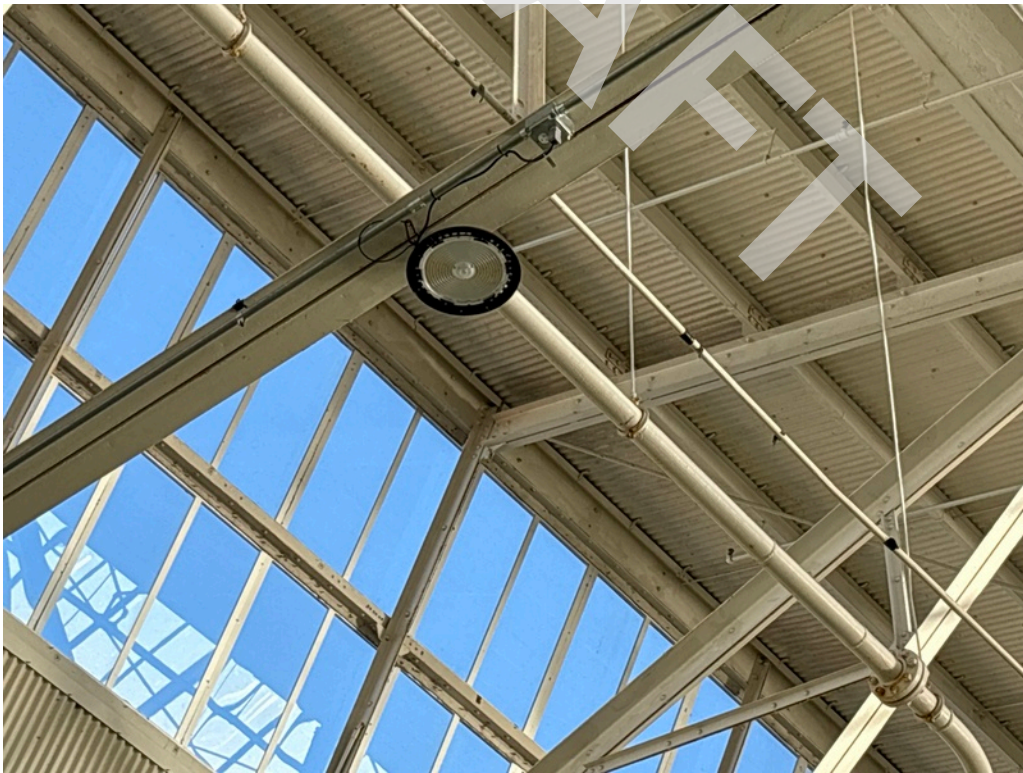
44 - Typical high-bay LED light fixture in the Craneway Pavilion.
