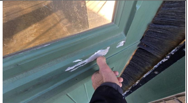
Figure 38. Paint failure on wood door frame
