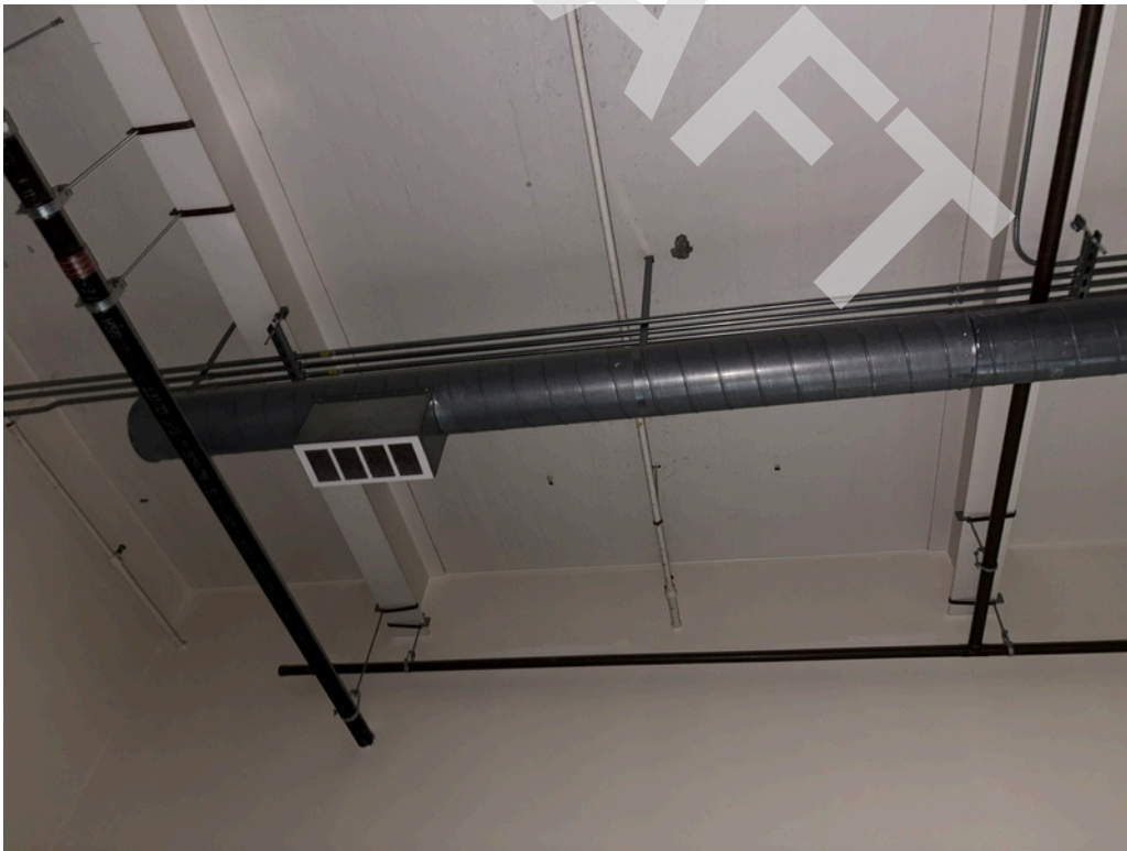
30 - Typical outside air supply ductwork and diffusers in the restroom.
