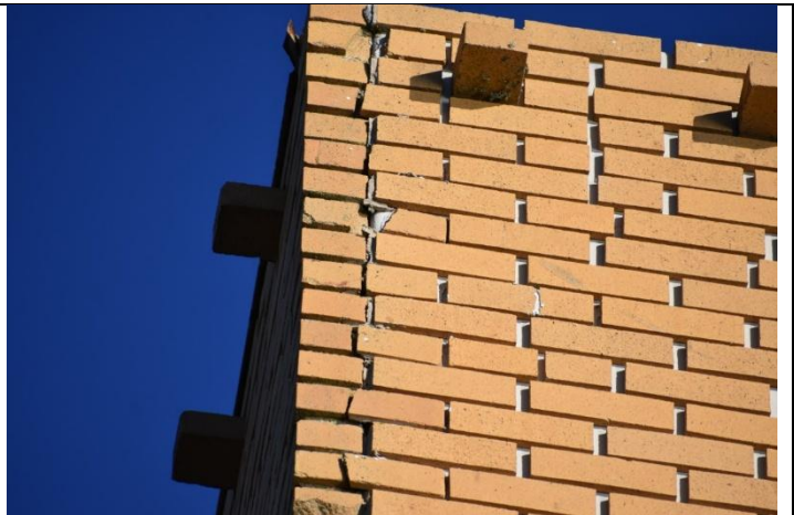
Figure 6. Vertical cracking at interface between brick masonry wall and FRP/fiberglass brick-veneer clad parapet at corner
