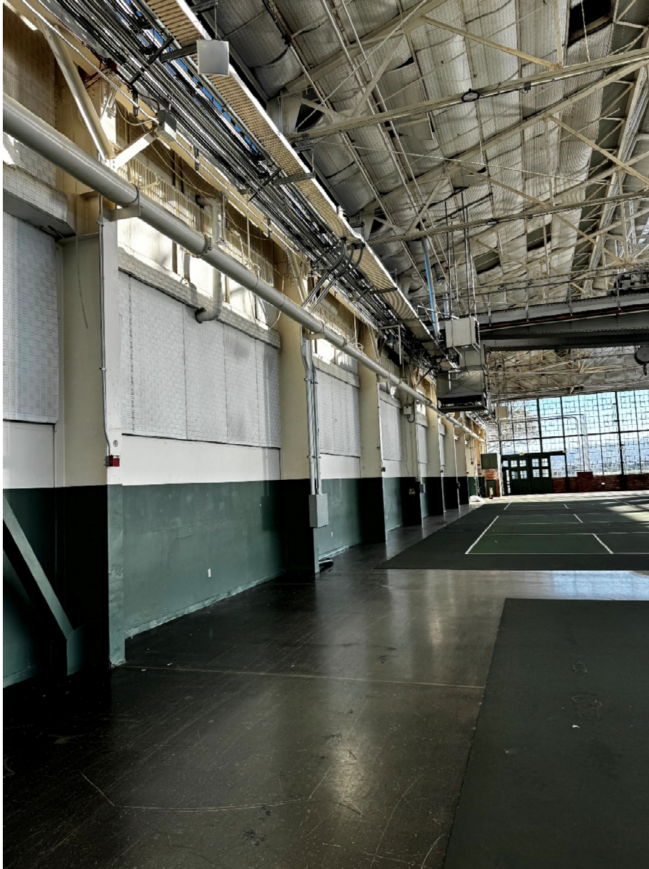
Photo 14: Interior piping tray and heater (1/8/2026)
