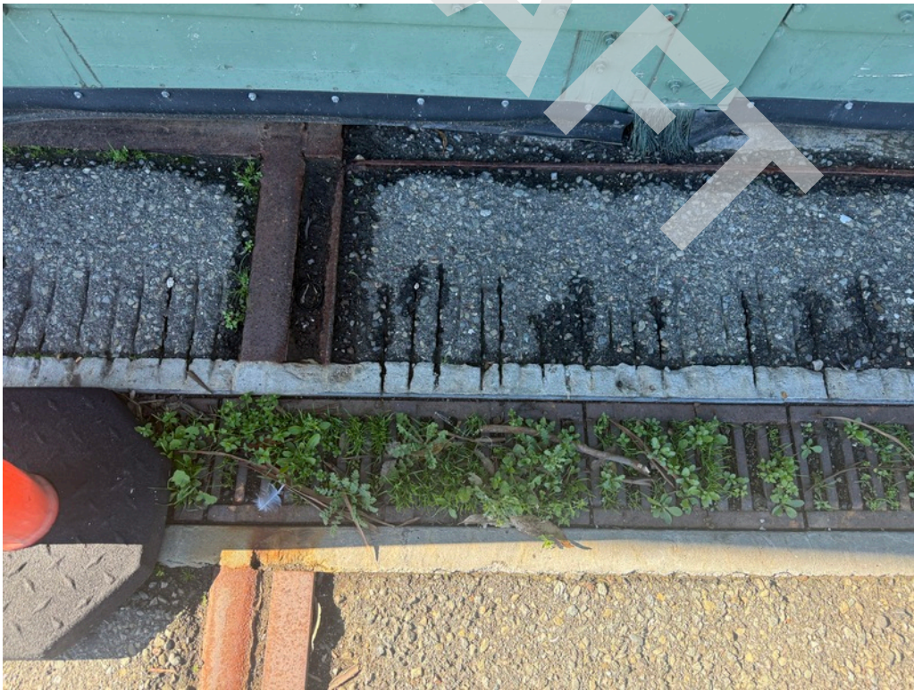
4 - Clogged trench drain along the east perimeter of the building.
