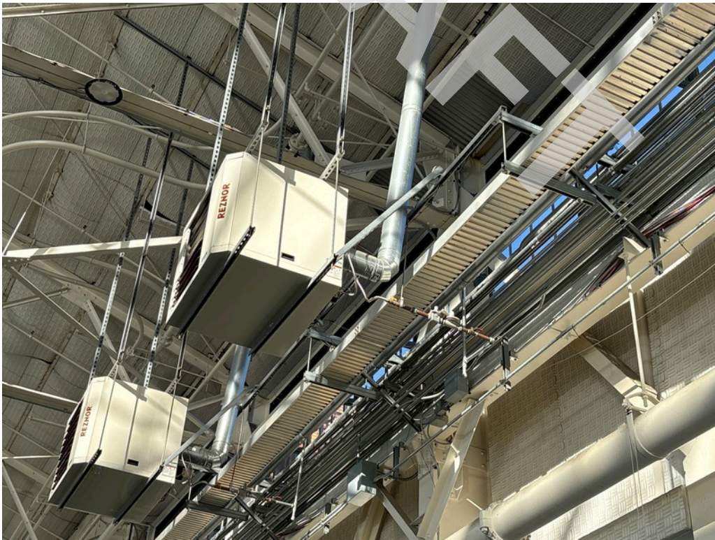
26 - Typical ceiling-hung unit heaters in the Craneway Pavilion.
