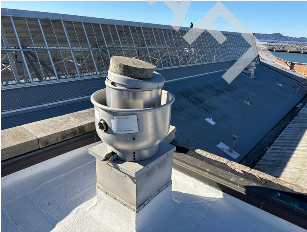
28 - Dishwasher exhaust fan on the roof of the small Main Building tower projecting above the main roof.
