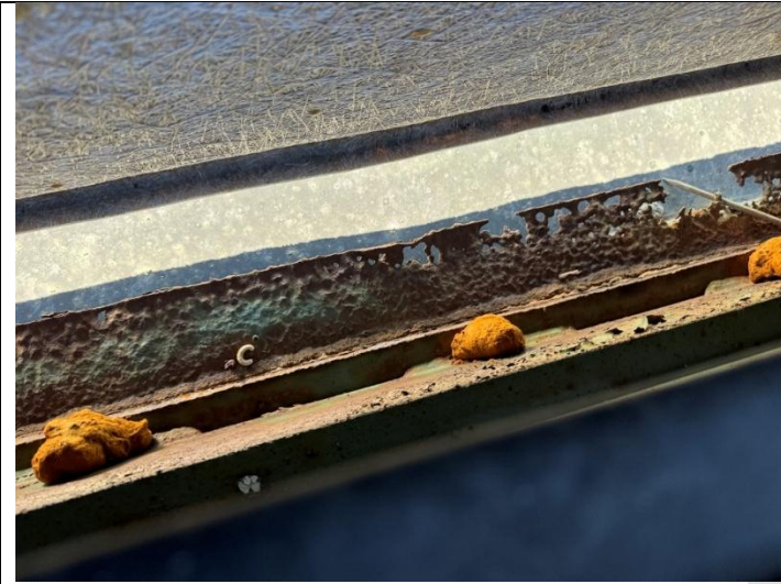
Figure 57. Significantly corroded steel angle behind base of newer parapet panelized cladding; likely abandoned
