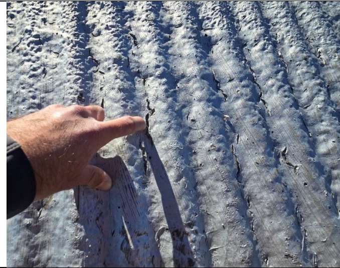
Figure 49. Failing coating over transite panels
