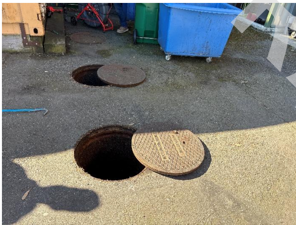
Grease trap north of the restaurant.
