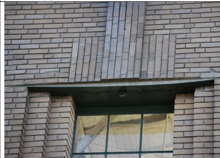
Figure 11. Deflection/sagging of brick lintel
