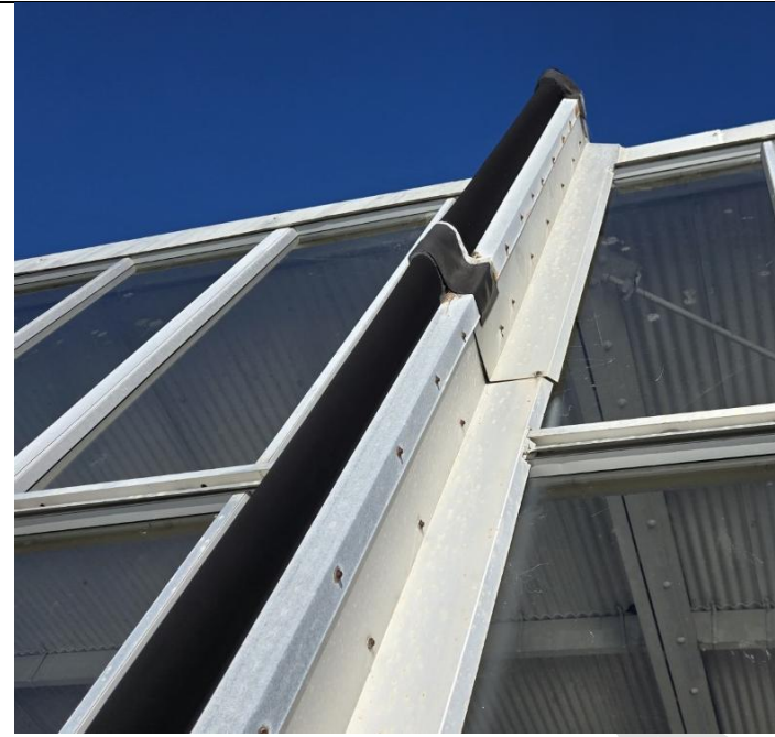
Figure 65. Expansion joint bellows transitioning across skylight assembly
