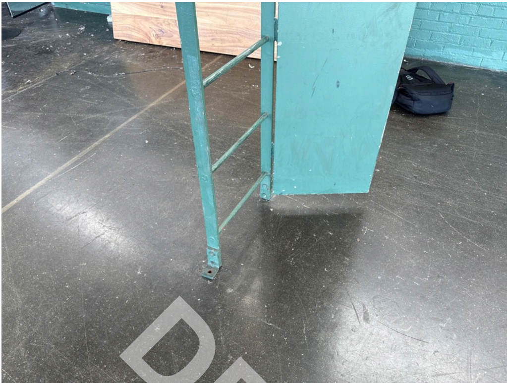
63 - Beam crane operator's station access ladder with missing bolt.
