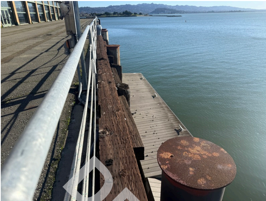
9 - Corroded steel piles at the main pier along the south perimeter of the site.
