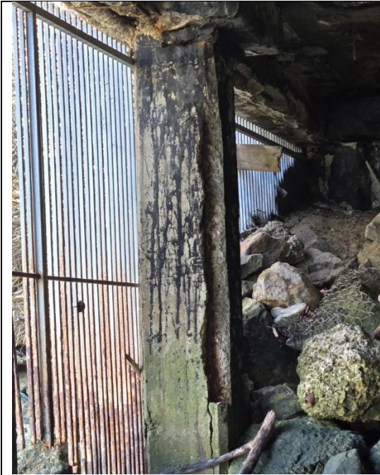
Figure 73. Significant spalling and sectional loss present, corroded reinforcing visible – Severe Defect Category
