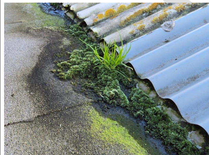
Figure 59. Organic material growth and ponding at low-spot near drains
