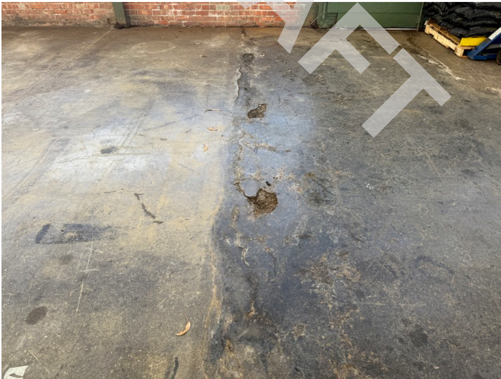
24 - Minor damage to the concrete flooring along the east elevation.
