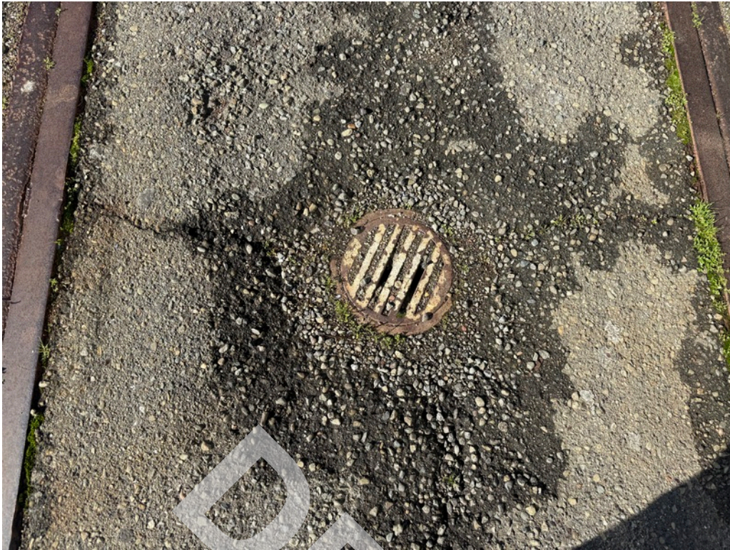
5 - Rusted area drain located along the south perimeter of the site.
