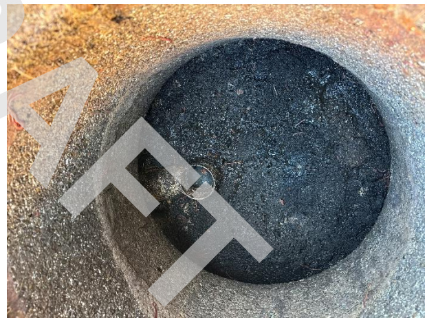
Discharge portion of the grease trap showing levels immediately below the rim of the pipe outlet (meant to flow only clear water).
