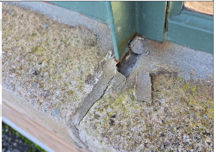
Figure 24. Failing mortar at window interface with stone sill
