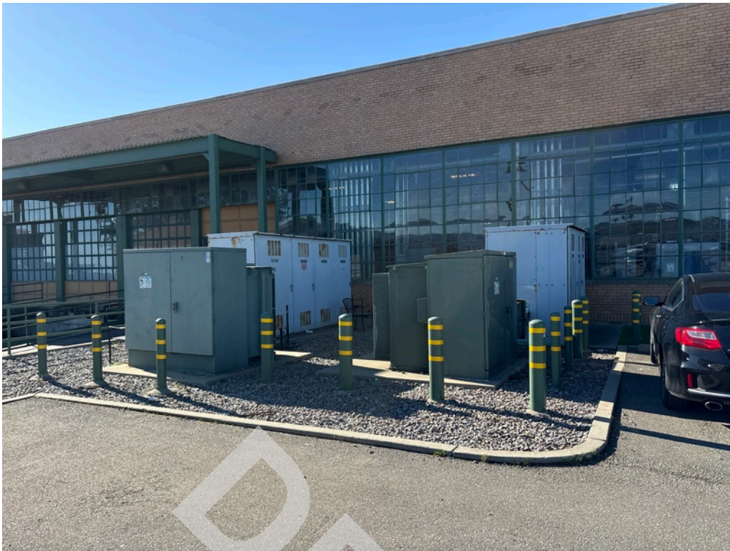
39 - Electrical yard on the southeast portion of the Main Building. One of these two transformers and termination cabinets serves the Craneway Pavilion.
