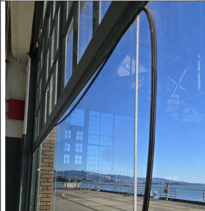
Figure 35. Disengaged gaskets at new butt-glazed window system on south elevation
