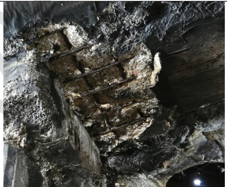
Figure 80. Sectional loss at underside of slab and corrosion of reinforcing steel
