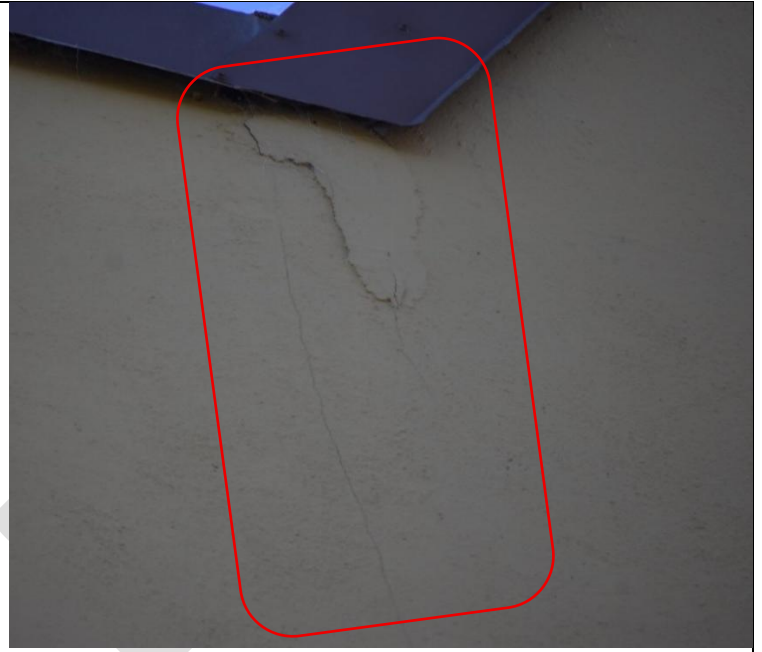
Figure 26. Vertical cracking through gunite wall
