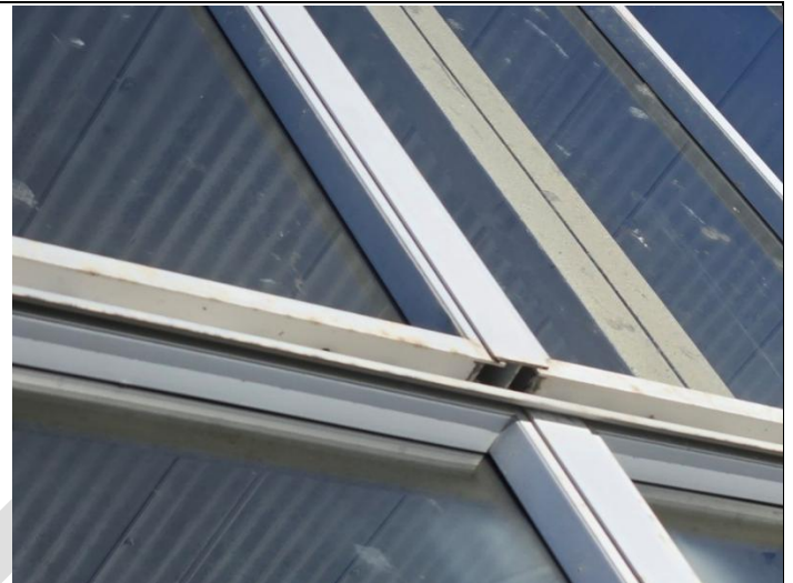
Figure 62. Skylight drainage at vertical mullions
