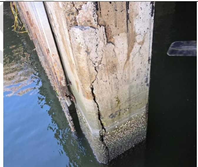
Figure 72. Significant spalling and sectional loss present – Severe Defect Category
