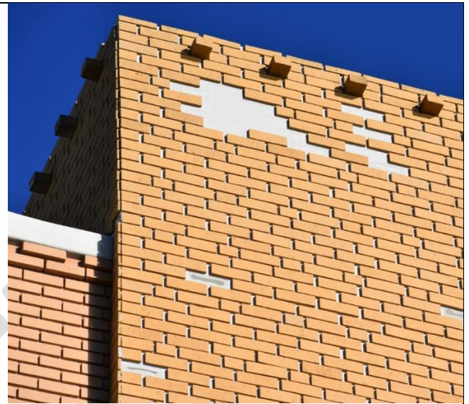
Figure 18. Missing brick veneer units
