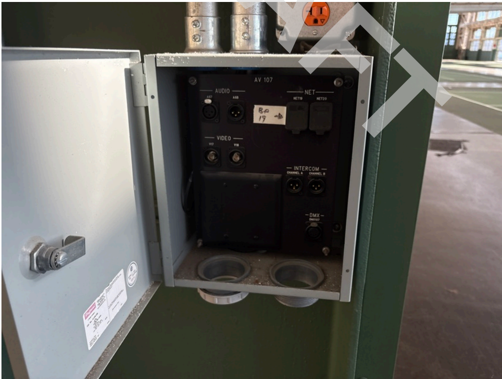
52 - Typical A/V system connection panel.
