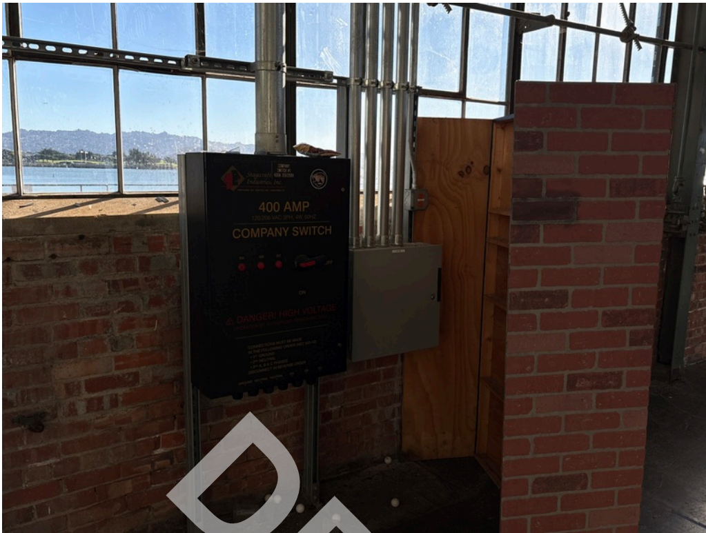
43 - The second of two A/V special electrical panels. This is located on the east wall of the Craneway Pavilion.
