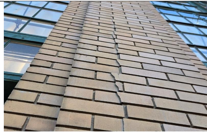
Figure 5. Vertical cracking and out-of-plane displacement at column on west elevation
