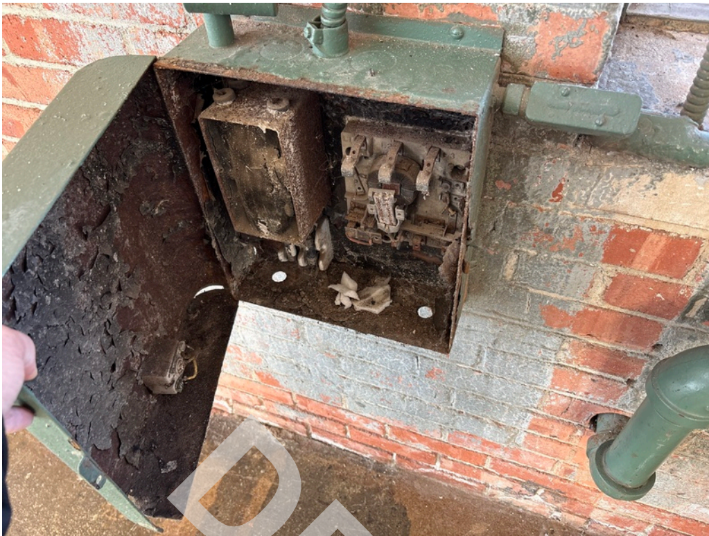
49 - Abandoned safety switch with damaged front cover on the west wall of the Craneway Pavilion.
