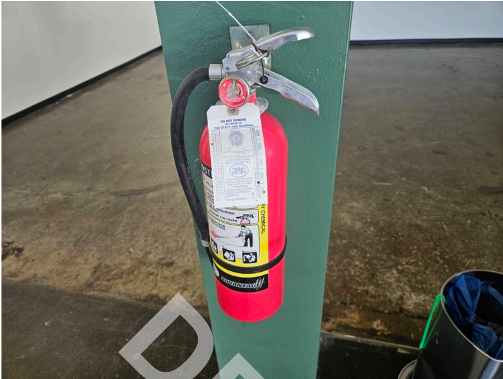
59 - Typical fire extinguisher.
