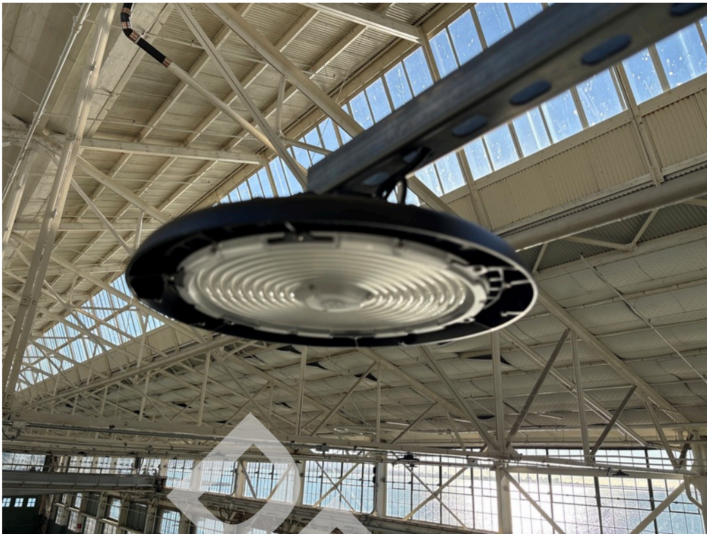
45 - Close-up view of typical high-bay LED light fixture.
