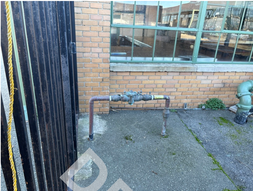
33 - Backflow preventer adjacent to the restaurant.
