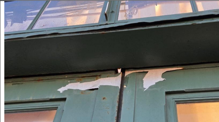
Figure 37. Corrosion and paint failure on original steel door frames
