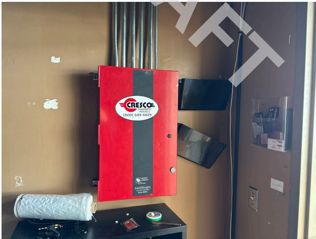
54 - Satellite fire alarm notification panel in the office/utility room of the Craneway Pavilion.
