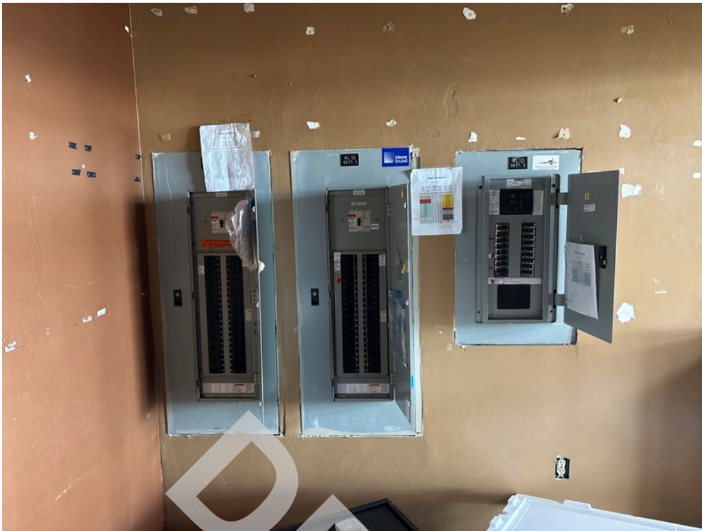
41 - Distribution panels in the Craneway Pavilion office/utility room.
