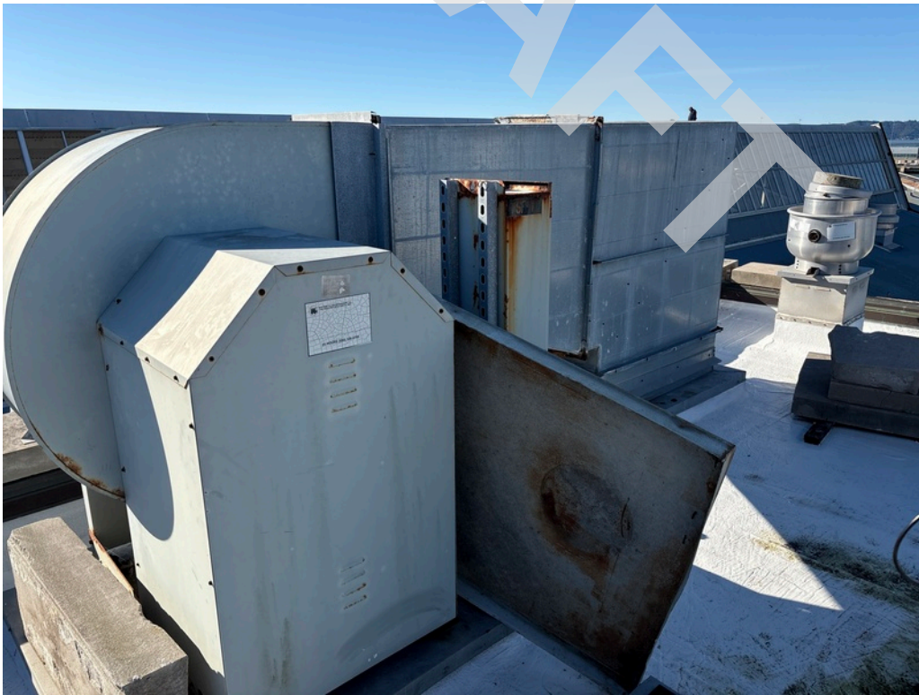
32 - Outside air supply fan for the service kitchen on the roof of the small Main Building tower projecting above the main roof.
