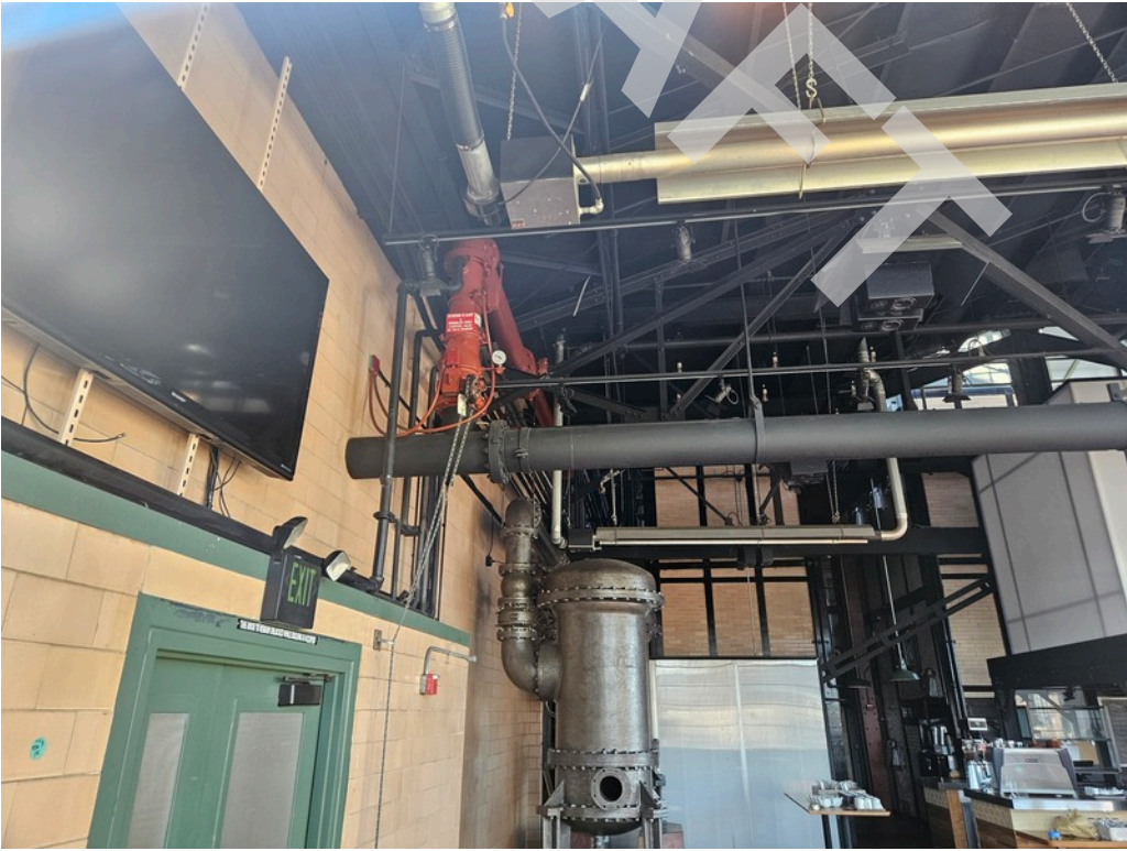
56 - East sprinkler riser.
