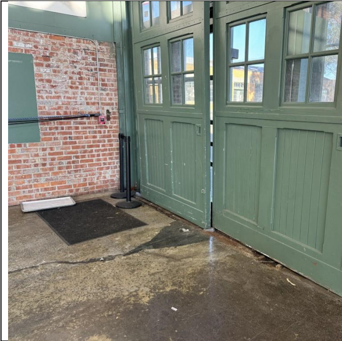
Figure 41. Gaps between adjacent door segments; not air and water tight
