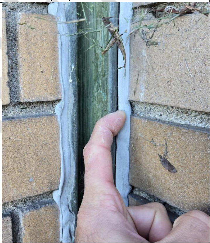
Figure 8. Sealant deterioration at vertical expansion joint on west elevation
