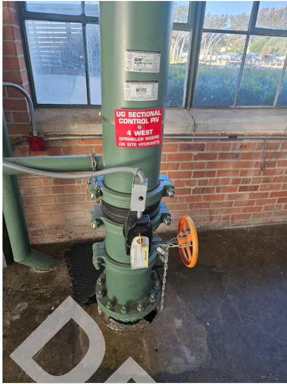
55 - West site water loop connection.
