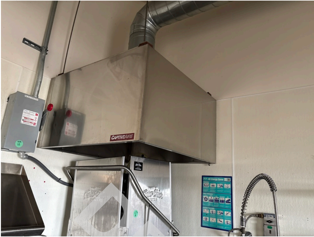
27 - Dishwasher exhaust hood in the service kitchen.
